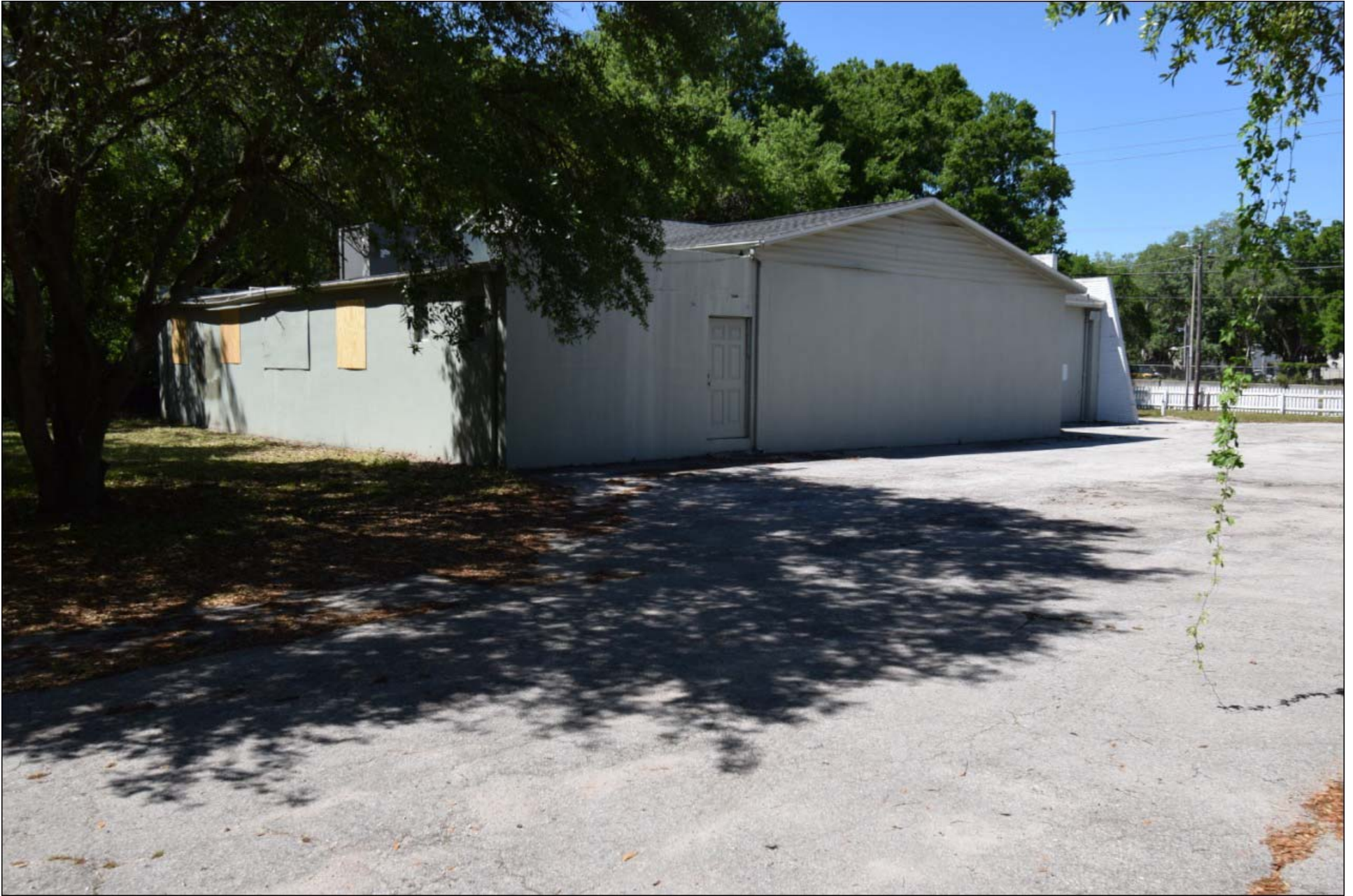
Back of Church – New 7 Ton A/C on roof
